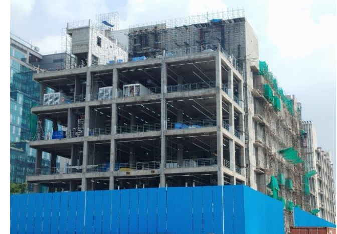
Mindspace Airoli West Building 8- Data center (~0.3 msf) Estimated Completion – Q4 FY25
