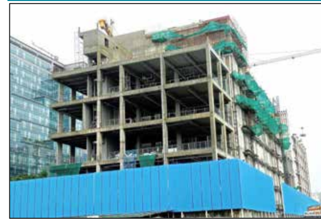
Mindspace Airoli West Building 8- Data center
